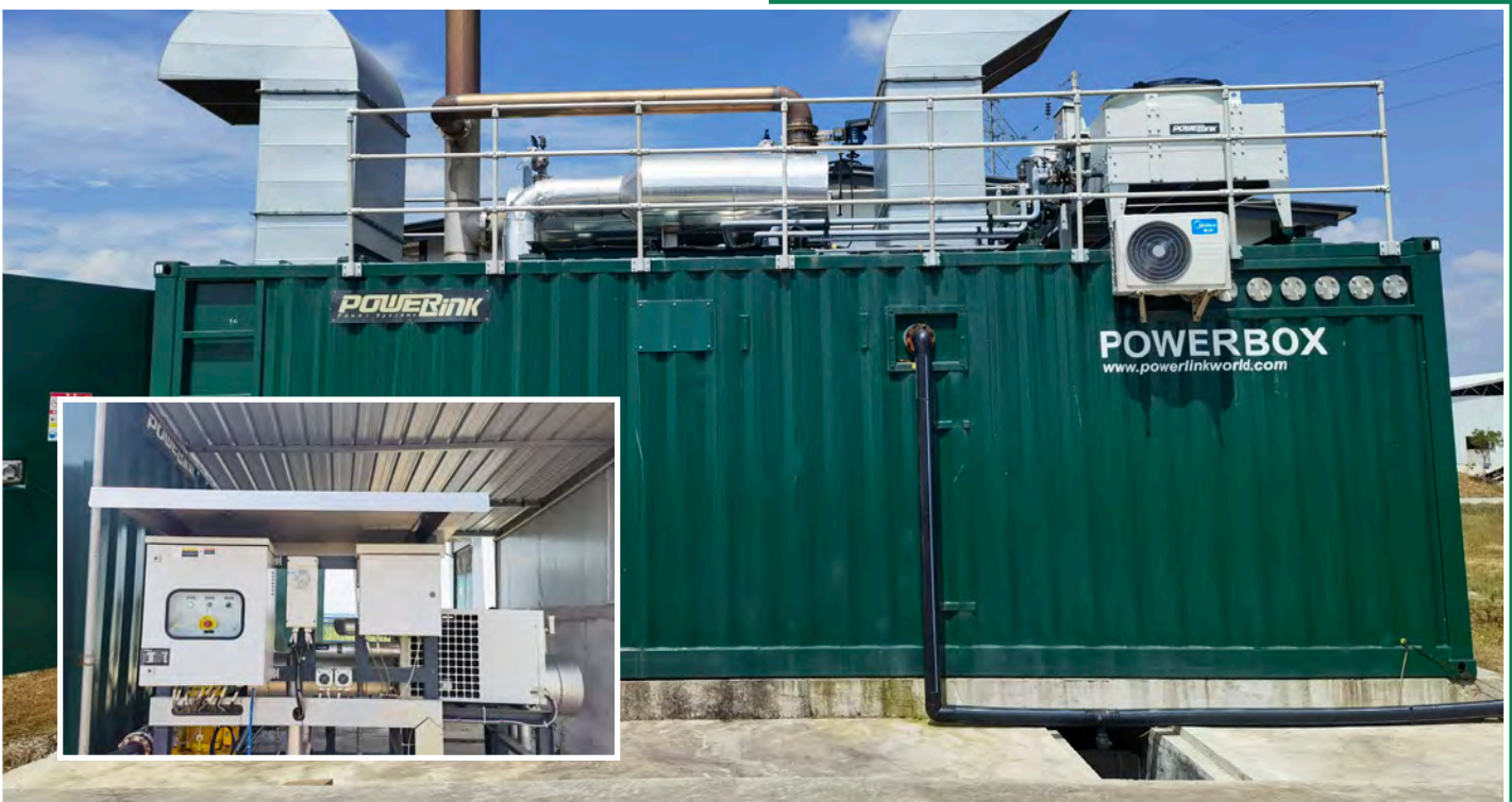
Farm Biogas Cogeneration Application 500KW
